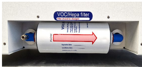
Figure 12.3 Correctly installed VOC/HEPA filter
